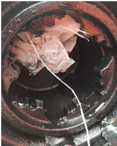
Figure 3-19: Debris pumped through
