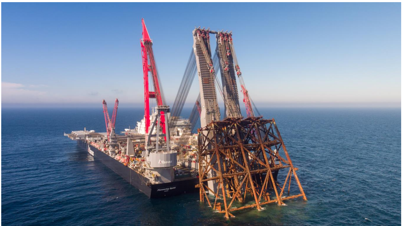
Pioneering Spirit removes the Ninian Northern jacket with its new Jacket lift system
