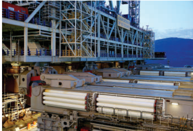
All yokes connected to the topsides.
