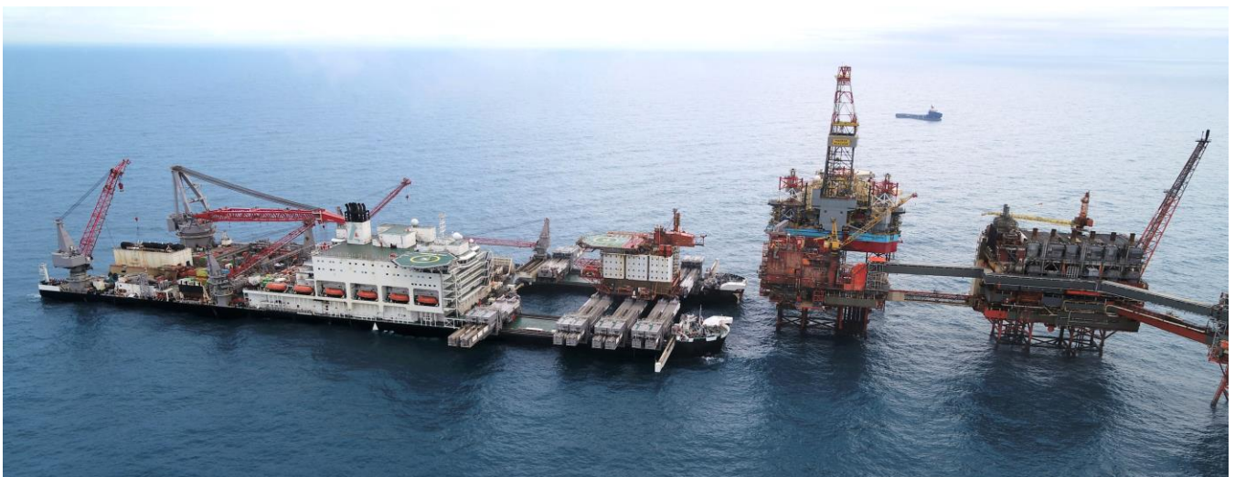
Pioneering Spirit safely removed the 3,800 t QP topsides in June 2019 and will return to remove the DP and PCP platforms and connecting bridges (pictured)
